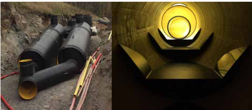
Figure 5. Step aerator built in Turku, Finland. The aerator was placed after a pressure sewer line and before a concrete gravity sewer. The first 400 m of the gravity sewer was coated at the same time, as there was a lot of concrete corrosion caused by H_2S . The flaps beside the steps allow the air inflow under the fall.
