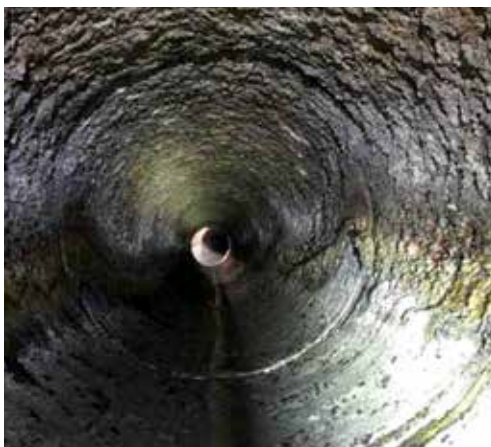
Figure 7. Raisio sewer line after 5 years' use. Concrete corrosion was caused by hydrogen sulphide.
