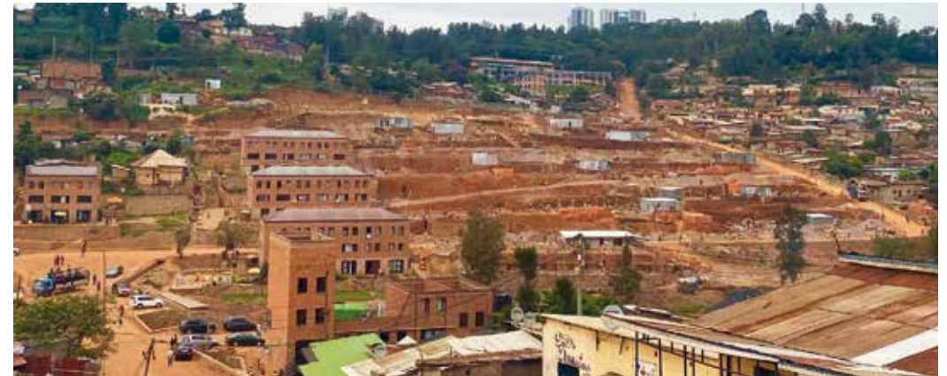
Figure 4. Removal of informal settlements and preparing the foundations of new blocks in Mpazi.
