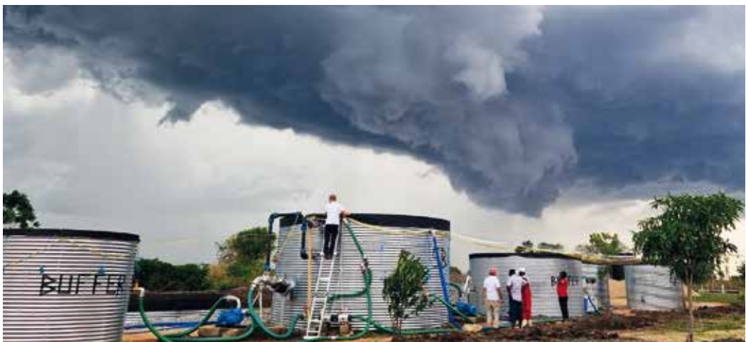
Figure 2. The Faecal Sludge Management Emergency Response Unit (FSM ERU) treatment plant piloted in Imvepi, Uganda, 2025 showing from left to right the solid-liquid separation (SLS); buffer tanks holding supernatant after sedimentation; the sequencing batch reactor (SBR); buffer tank before hygienisation; and behind the SBR the sludge drying beds (SDB).
